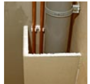
Very simple covering of pipes and drains.
